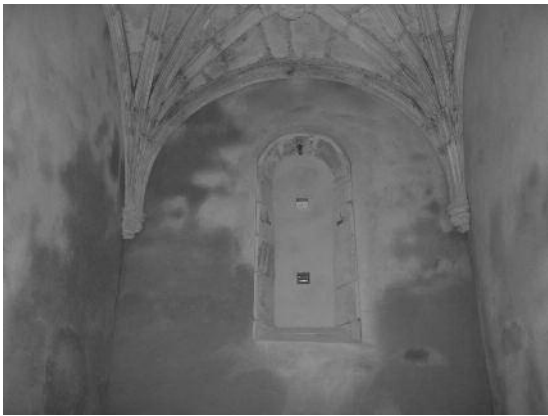
Fig. 4 Drying of a lime-base rendering inside a church in Northern Portugal (September 2004 and January 2005).
